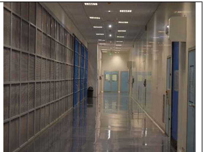
Cleanroom walls, ceiling and view panels installed in a warehouse along with epoxy flooring
