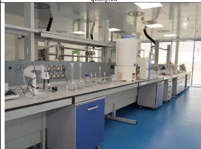
Designed, procured and installed lab furniture along with lab equipment as part of the turnkey project
