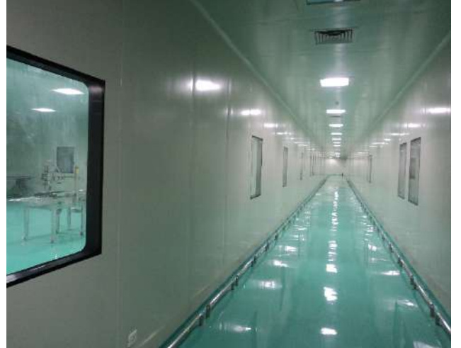
Facility corridor where cleanroom walls, ceiling and view panels have been installed along with epoxy flooring
