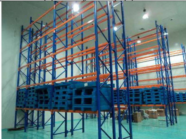
Installed warehouse rack with pallets
