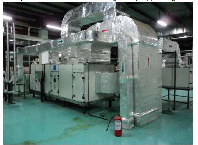
Installed air conditioning systems in the entire facility
