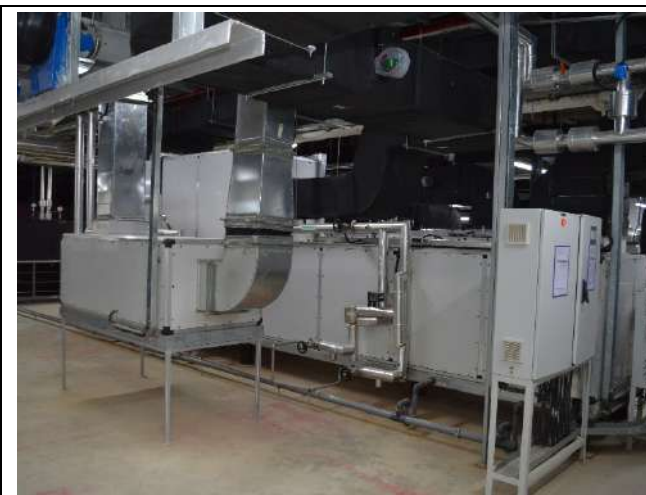
Air handling unit supplied and installed, commission and qualified
