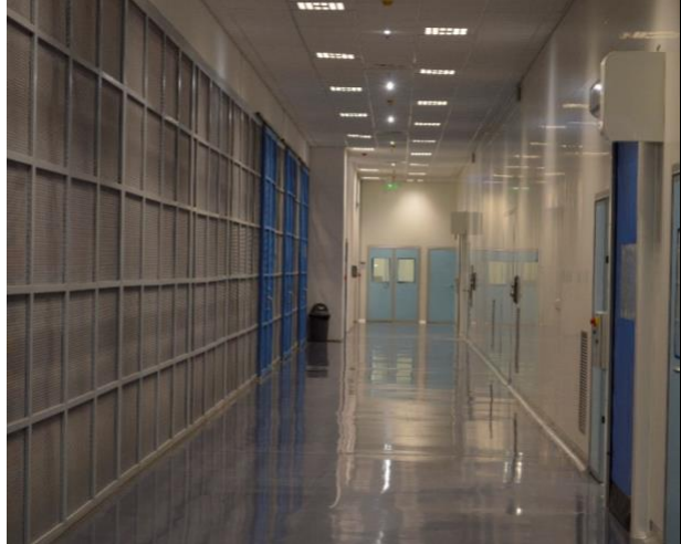
Cleanroom walls, ceiling and view panels installed in a warehouse along with epoxy flooring
