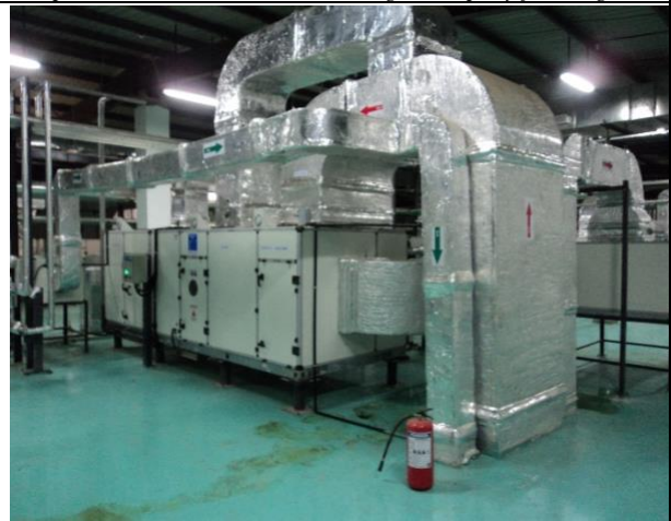
Installed air conditioning systems in the entire facility
