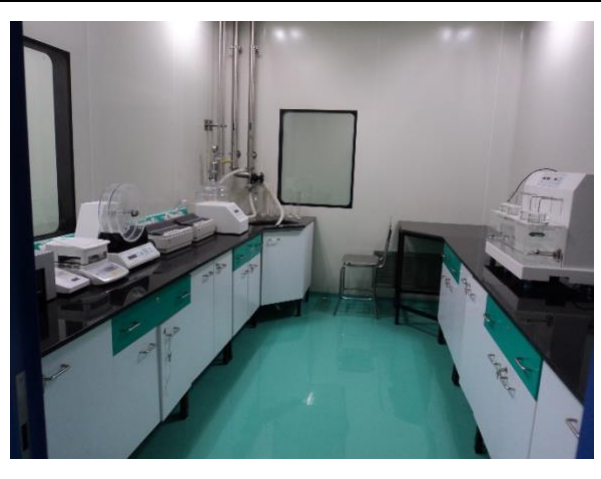
Designed, procured and installed lab furniture with lab equipment, as part of the turnkey project
