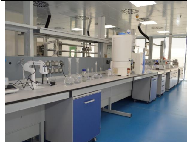
Designed, procured and installed lab furniture along with lab equipment as part of the turnkey project
