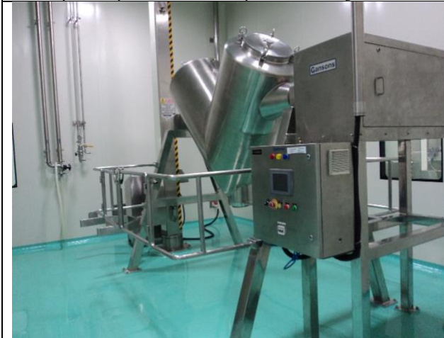
Supplied, installed, commissioned and calibrated manufacturing equipment along with utility equipment
